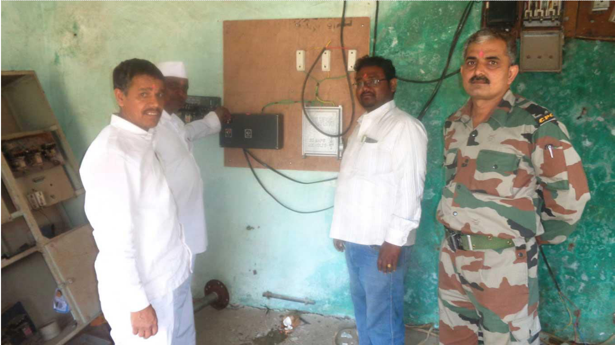
INSTALLATION OF PUMP & PIPE LINE FOR SUPPLY OF WATER TO TALEGAON, ANJINARI, NASHIK.
